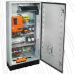
Pano Control panel
